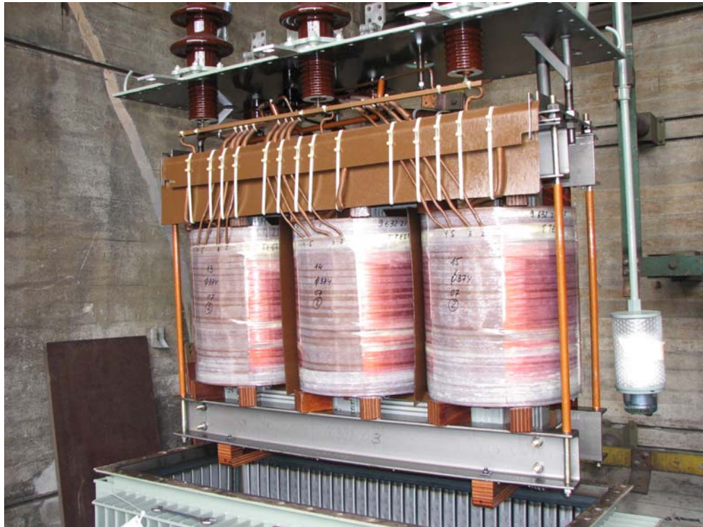
Fig. 3 Active part of tested transformer (HV-terminal side) after all tests
