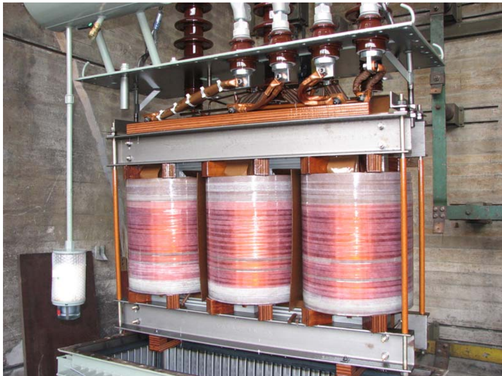
Fig. 4 Active part of tested transformer (LV-terminal side) after all tests
