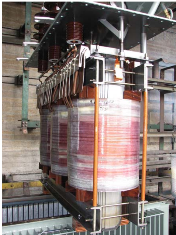
Fig. 6 Side view (phase C) of active part after all tests
